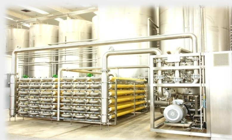
● RO Water treatment UF 4, 20T/H
